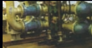
PUMPS / VALVES POWER GENERATING
