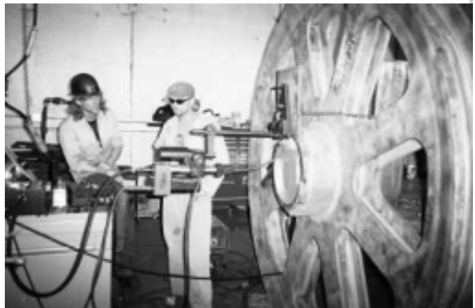
Here a large flywheel is repaired with a Bortech unit. Not only saving money but actually improving versus using a bushing type repair.
